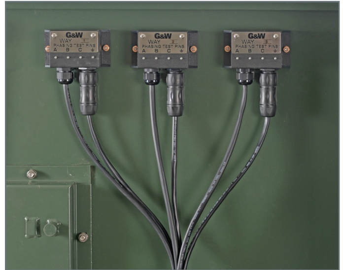
▲ Voltage Phasing Test Pins installed on a padmount enclosure.
