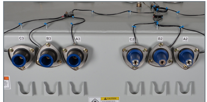
▲ Voltage sensing bushings mounted on a G&W SF6 insulated switch.
