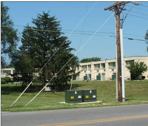
Each of two separate circuits were terminated into padmount enclosures located adjacent to each other.
