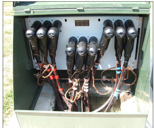
Sectionalizing cabinet incorporating three, 600A, 3-position junction bars.
