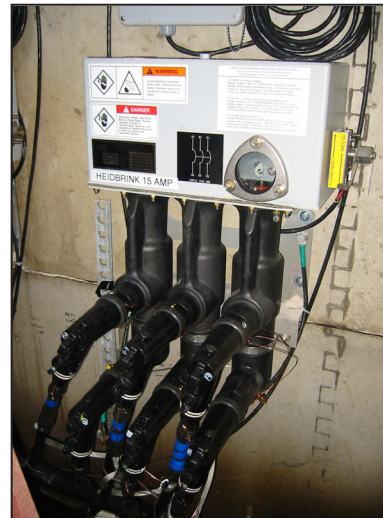
Figure 2: Three phase interrupter mounted to vault wall. Operating handle permits manual reset of all three phases. and is accessible from above ground using a hookstick.
