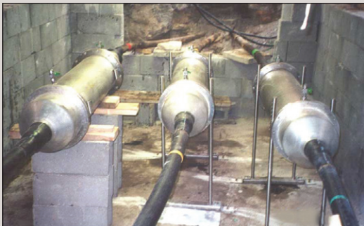
Distribution Cable Joints
