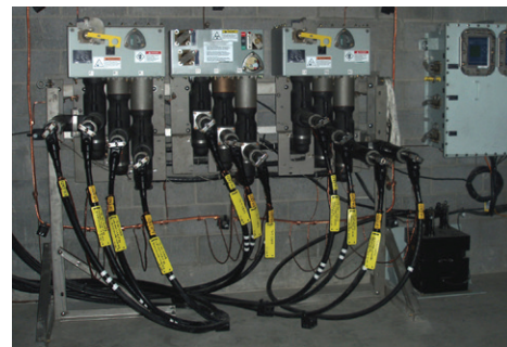
Solid Dielectric Vault
